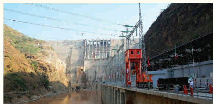
The AfDB has assisted with numerous interconnection projects to improve regional power infrastructure
